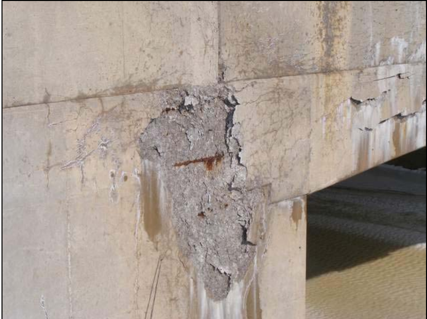
Figure 5 - Deterioration at West Wingwall and Haunch
