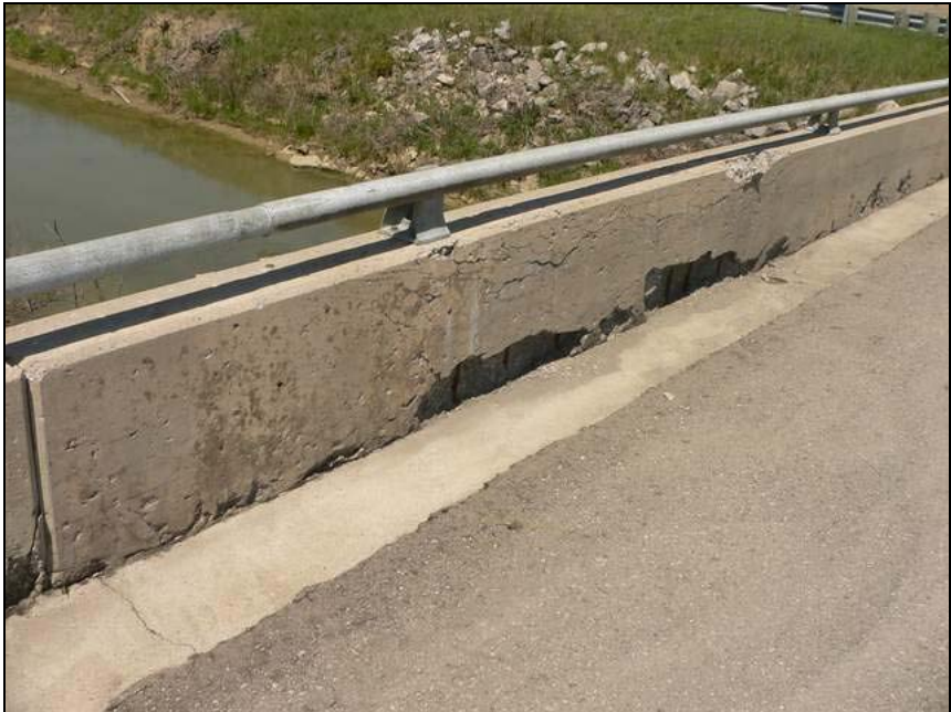
Figure 3 - Deterioration at North Parapet Wall
