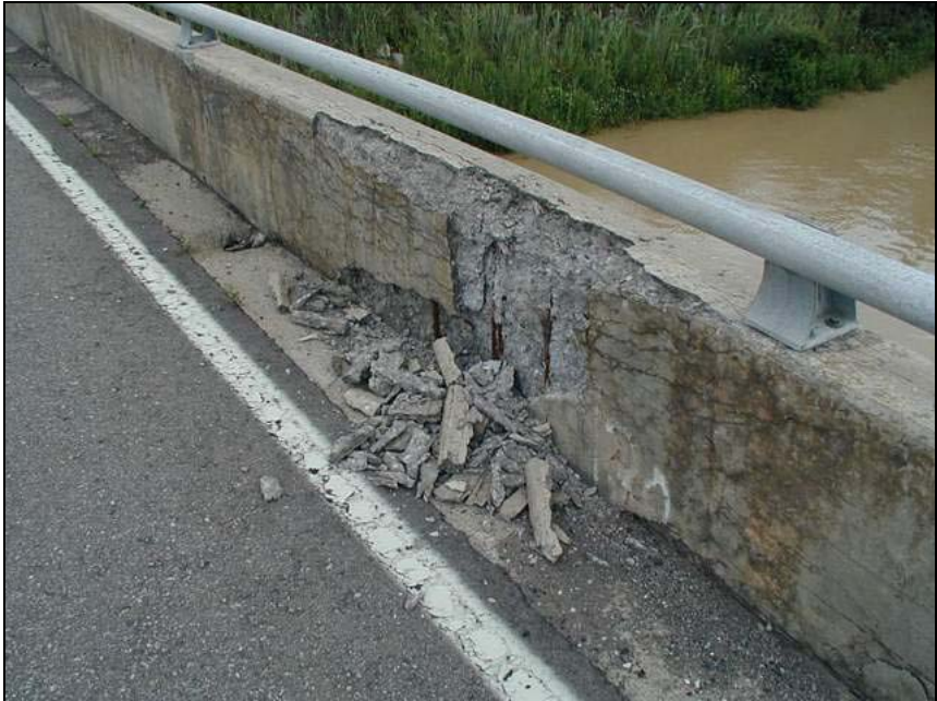
Figure 4 - Deterioration at South Parapet Wall
