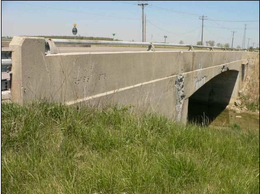
Figure 6 - Deterioration at South Elevation of Structure
