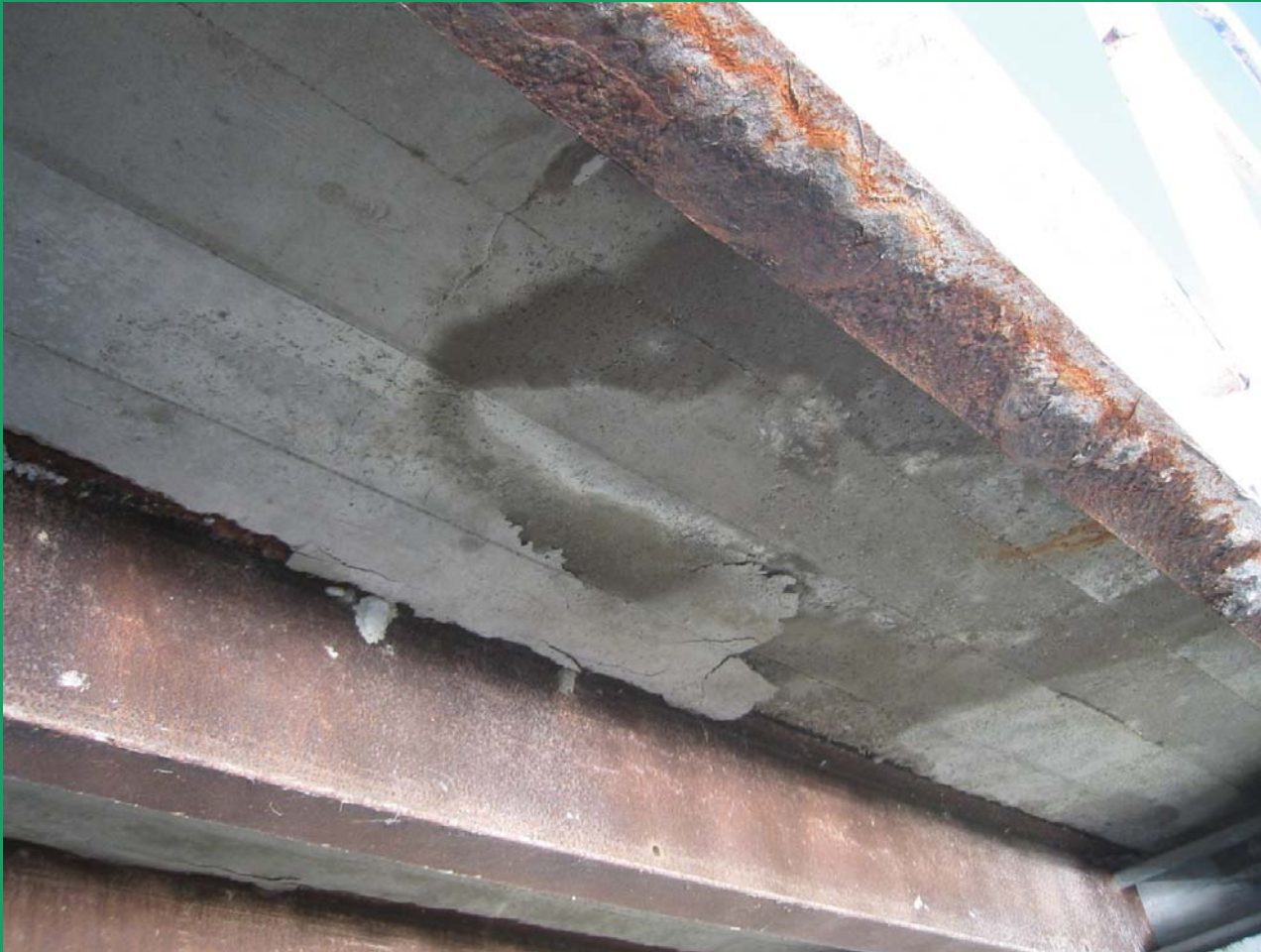
Delamination Underside of Deck
